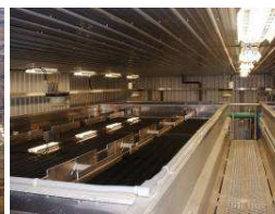
Joint Use Water Treatment Facility
