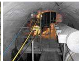
Sludge Line Twinning
