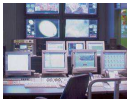
Airport Operations Control Center
