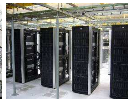
Data Center Independent Design Review
