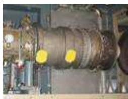
6 MW Cogeneration Plant Expansion
