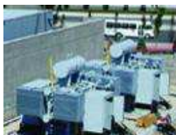
44 kV Airport Cogeneration Substation
