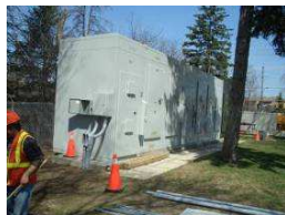
Pharmaceutical Company - Cogeneration Plant and High Voltage System Upgrade
