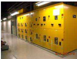
Internet Data Centre for National Telecommunications Company
