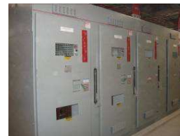
High Voltage Power Distribution for an Educational Institution
